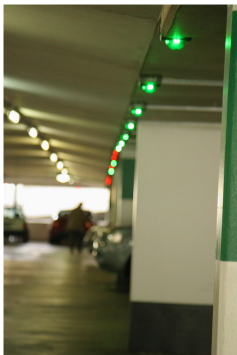
Parking guidance at Canberra Centre (QIC)
